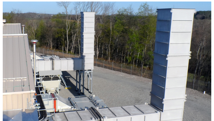
Turbine ducting systems
