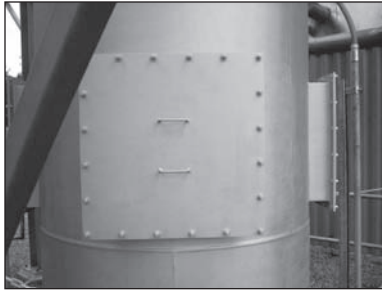
Figure 2: Proper positioning of catalyst access doors at the site is important for easy service.
