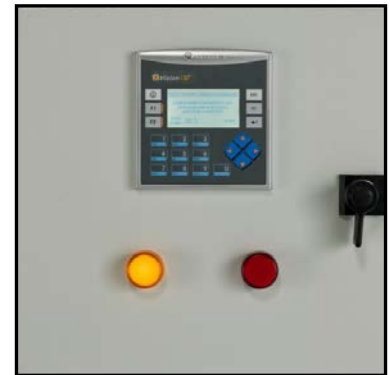
The GreenShield Catalyst Monitor provides data logging, text readouts and color-coded visual alarms.
