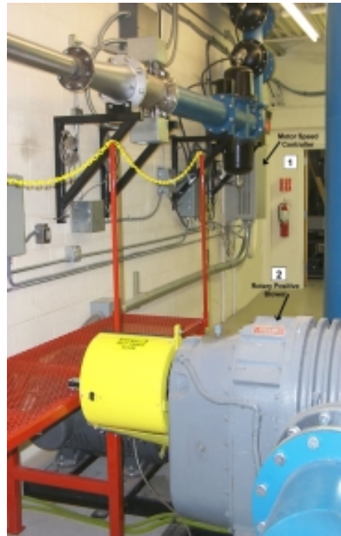
Figure 2 - View showing motor, controller and RPD blower
