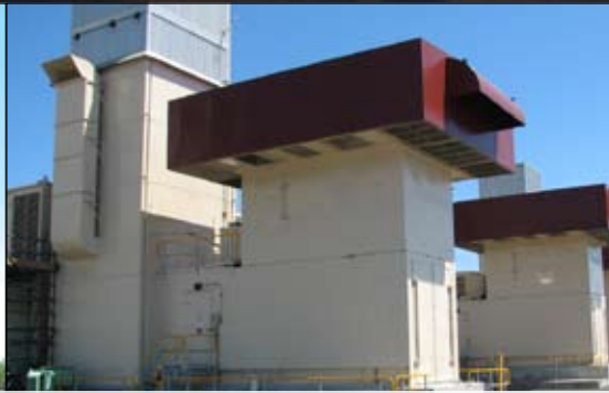
Inlet filtration and silencing
